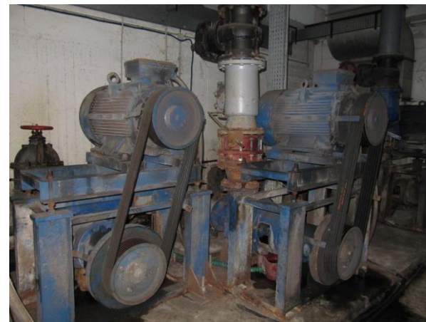
Pumps in Agia Fotini pumping station, Rethymno
